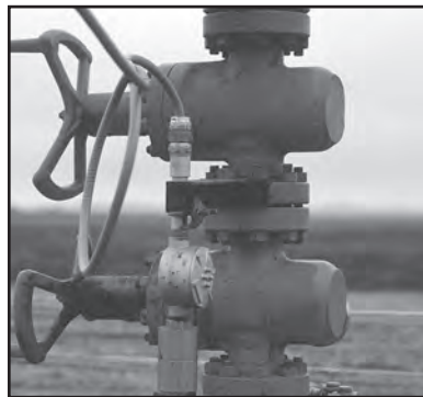
Wellhead and gas detector.
