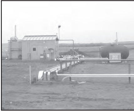
Process buildings may require permanently installed gas monitors to achieve Zone 2 classification.
