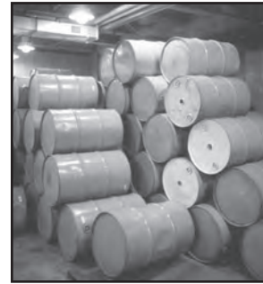
Areas where volatile liquids are stored are normally classified as Zone 2 or Division 2.
