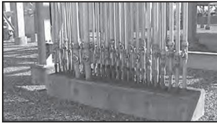
Seals are required when conduit leaves a Zone 1 area.
